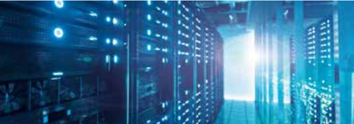
Emergency Power, UPS and CPS Systems
